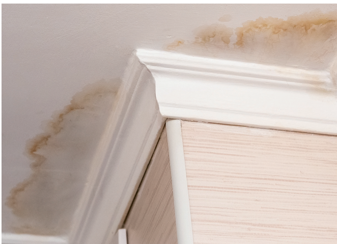
Condensation mould forms on ceilings when moisture laden air condenses on a cold surface.
